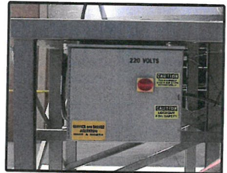
Electrical control panel and agitator timer is enclosed within a single weatherproof NEMA 3R enclosure.
