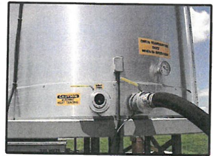
Heated & Insulated ball valves at the base of tank gravity feed emulsion to the Total Patcher.
