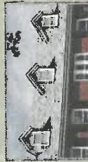
Slate roof restoration. Fabrication of new copper flashings & slate repairs. (Blue Forest, IL)
