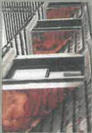
Complete restoration of clay roof, fabrication and installation of new copper gutters and flashings. (Providence St. Mel School)
