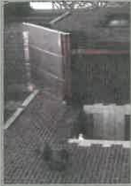
New standing seam copper bay roof, copper gutter and copper downspout below slate roof. (Darien, IL)
