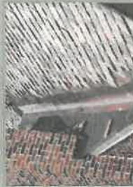
In the process of replacing copper valley flashing on slate roof and replacing slate roof. (Franklin Park, IL)
