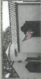
New and shiny tile roof installation. New copper and gutter flashings. (Skidmore, IL)
