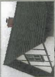
New green glazed French clay tile roof and new copper flashings. (Joliet, IL)
